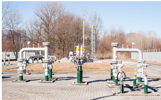
Natural Gas Pumping Station
